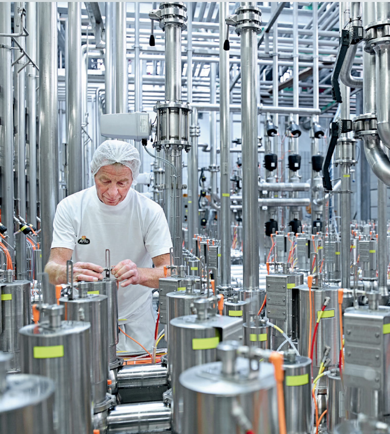
New frequency converter cut a third of the electricity bill, Denmark. Dairies in Denmark focus on efficiency. In one year, the Scandinavian dairy company Arla Foods saved nearly EUR 400,000 on its electricity bills for cooling towers by creating intelligent control of compressors and blowers by implementing Siemens' frequency converter. The payback time for the investment was just six months. (Courtesy: Siemens)
